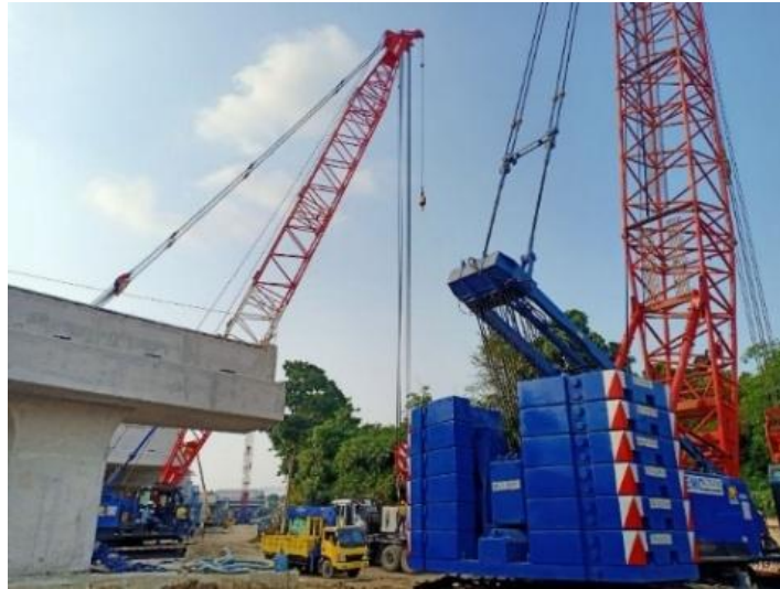
Gambar 2 Alat Berat Crane Crawler Sumber: Data Peneliti, 2025
